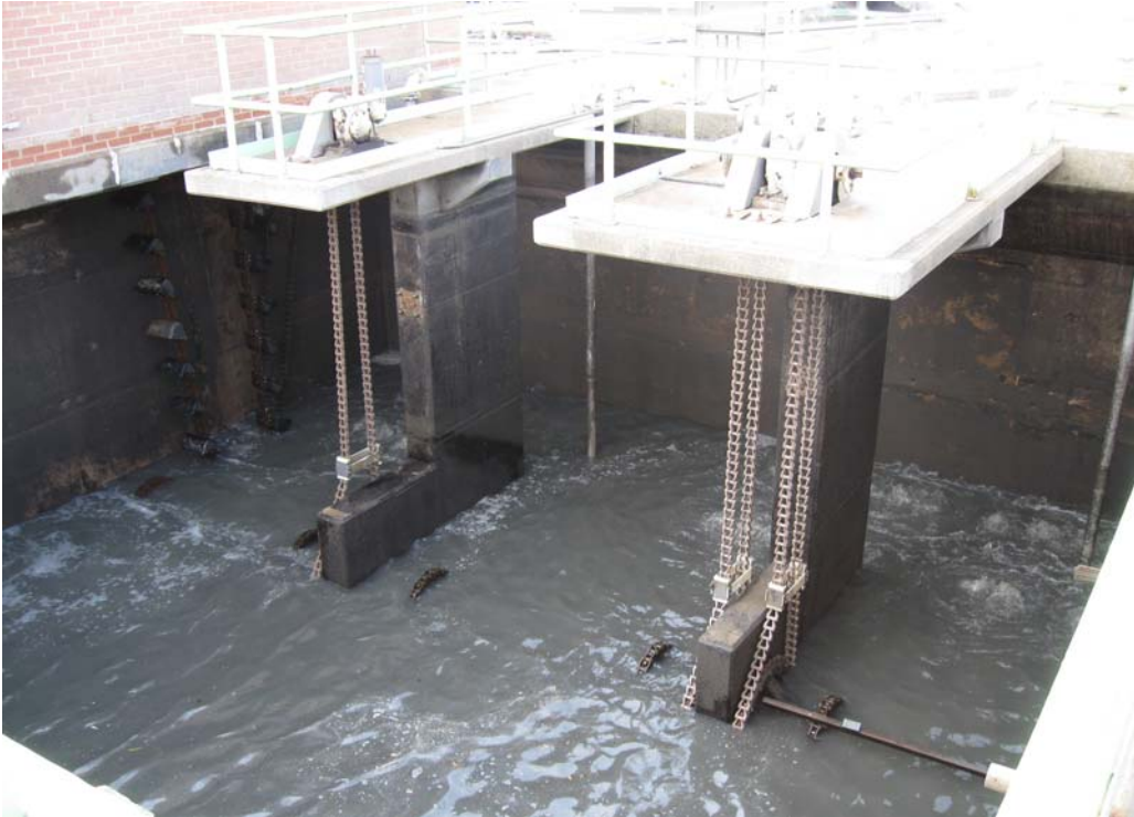
Figure 1 – Existing Aerated Grit Basin with Lowered Liquid Level
