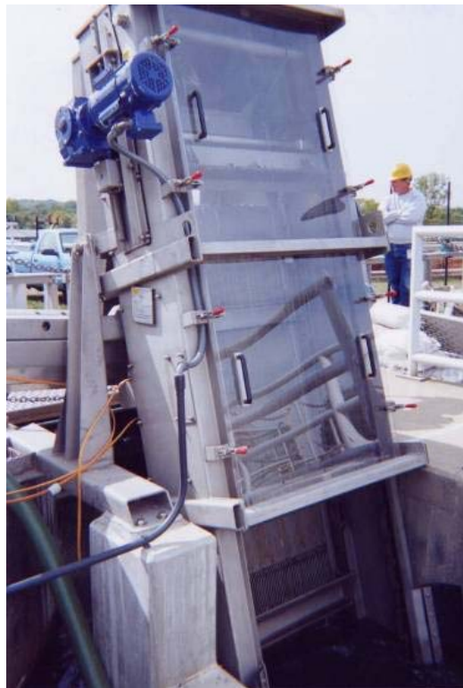
Figure 8 – Front Cleaned Bar Rack
