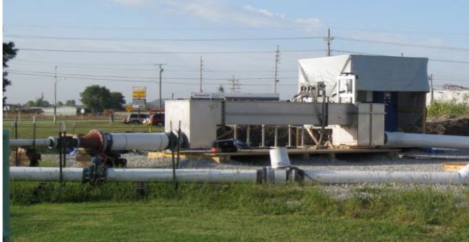
Figure 12 WEDECO UV Pilot Unit
