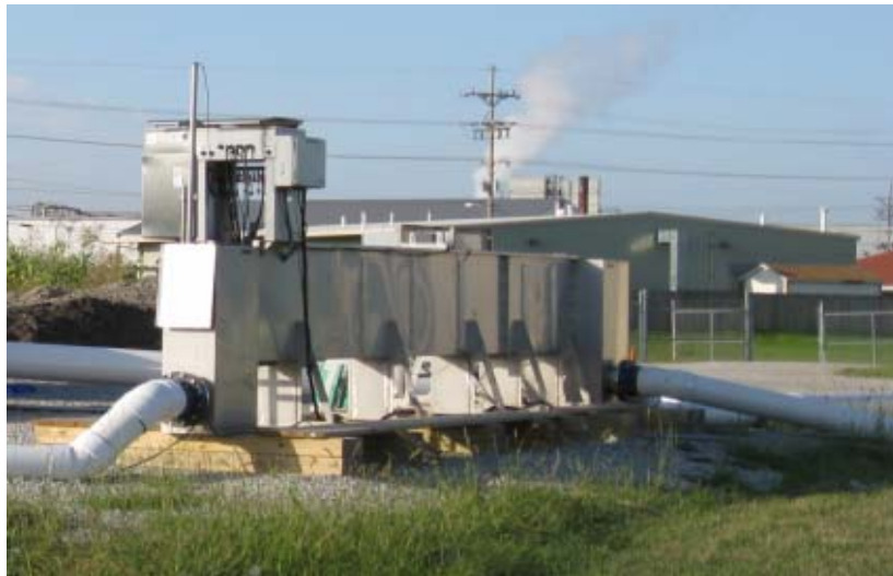
Figure 7 Trojan 3000Plus UV Pilot Unit
